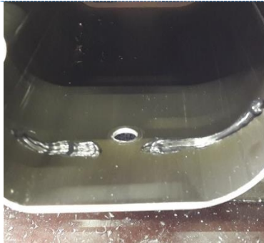
C. Clean the surface and put sikaflex or puraflex in front of the hole for the beambolt.
